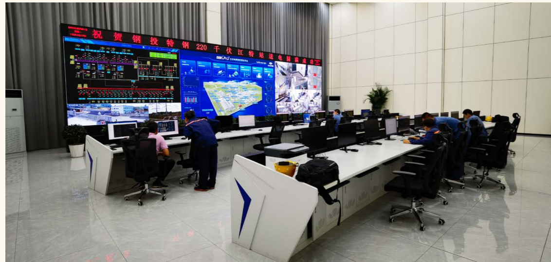
Enterprise power grid monitoring system
